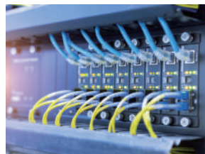
網路設備 Networking Equipment
